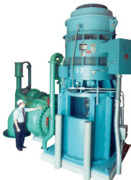
Figure 4. Floway 2500 HP - 900 RPM High Service Pump - Rigid Structure with 1st RCF above 1150 CPM.
