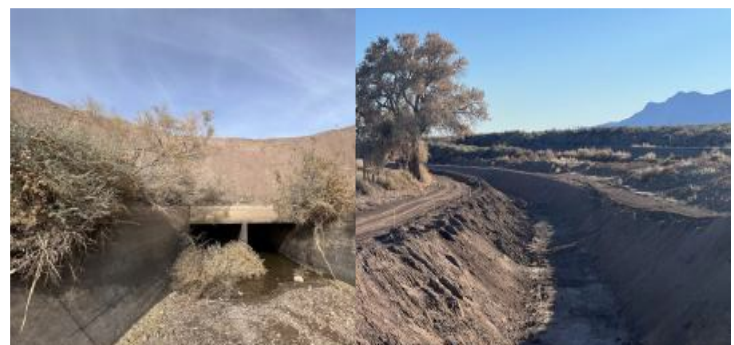
Figure 1. Vegetation damage to the canal and condition of the canal prior to final earthwork preparation.
