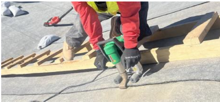
Figure 3: Ladders were used on long slopes to allow construction personnel to safely thermally bond the material and install the screws.
