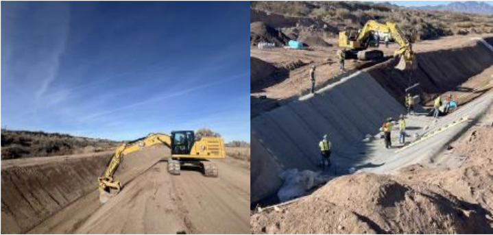
Figure 2: Subgrade being compacted and profiled for installation of GCCM and deployment of first rolls of GCCM into the canal.
